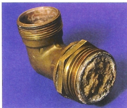
Example of severe limescale build-up
